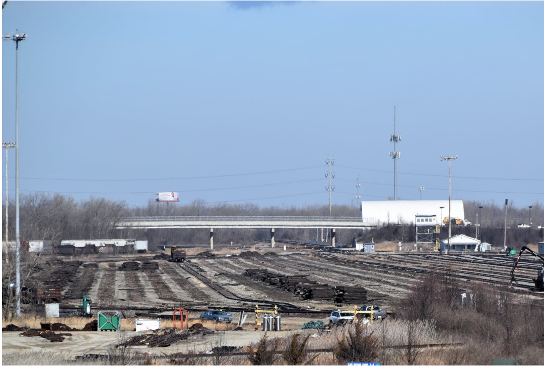
2021 – The heart of Buckeye Yard, the Classification Yard, is being taken up. Photo by Kenton Loy.
